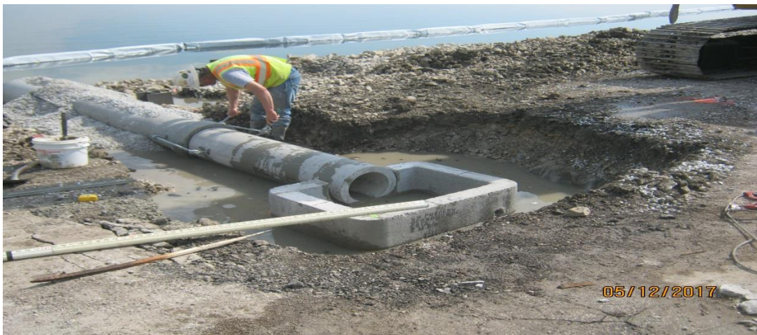
Installing reinforced concrete storm sewer that will run under the boardwalk and provide drainage for the parking lot.
