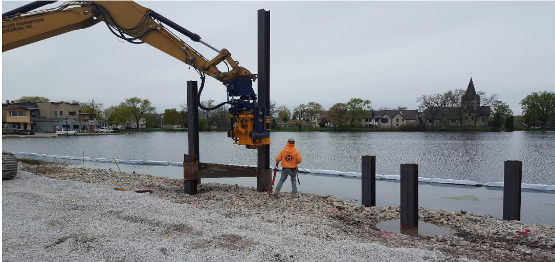
Piles being installed. The two piles closest to the Lake support the bumpouts while the pile further inland will support the boardwalk. The 25' long piles will anchor the boardwalk deep underground.
