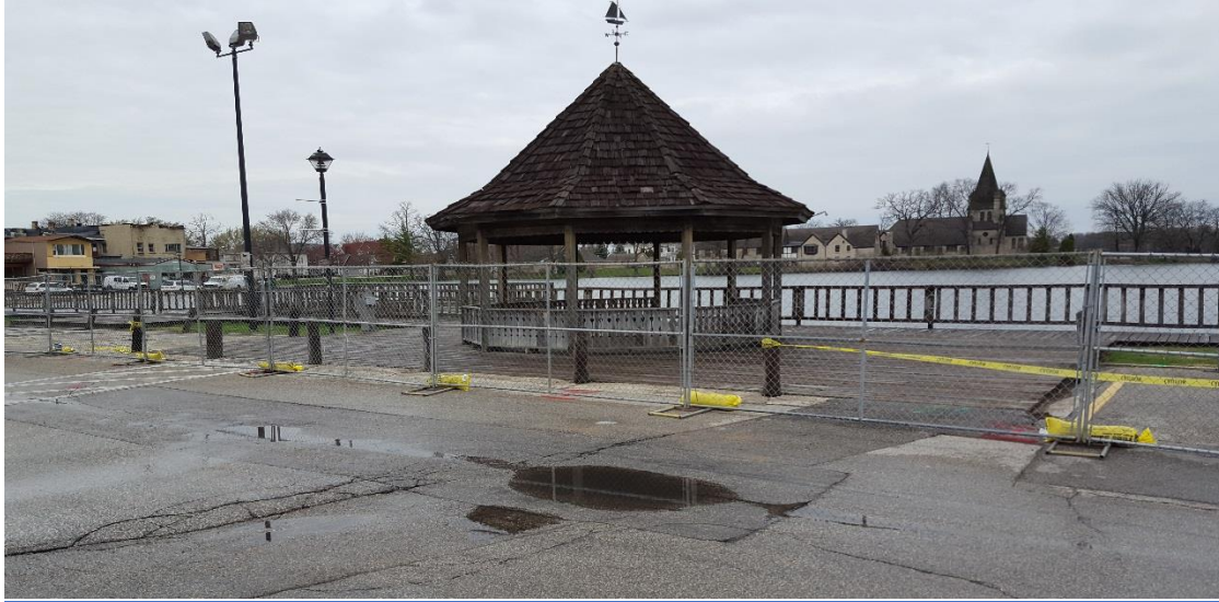
Fencing around the boardwalk project protects the safety of people in the area.
