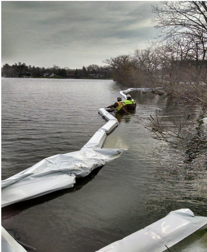
Installation of the Turbidity Barrier that is about 5' deep. The barrier prevents sediment during construction from entering the Lake. This protects water quality and lake habitat.
